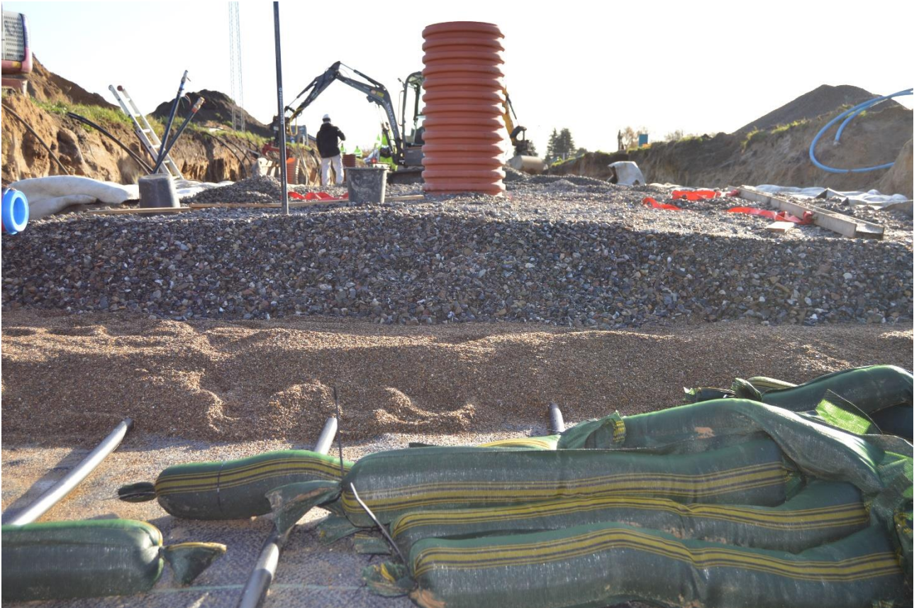
Figure 22. Ø40 mm SDR 11 geothermal U-pipe HEs buried in DrænAF soft gravel. The DrænAF is overlain by approximately 100 cm of DrænStabil coarse gravel.
