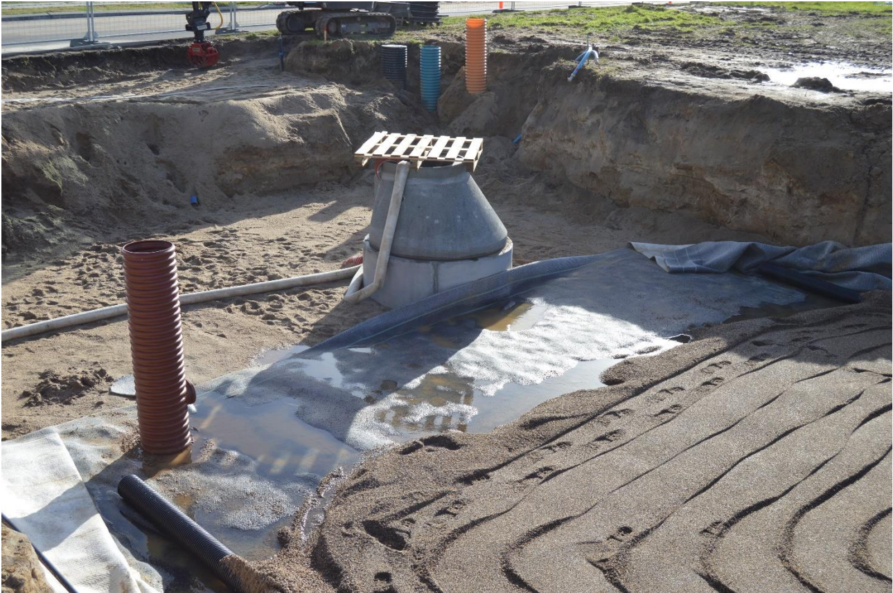
Figure 21. The concrete manhole containing the water brake is in the center of the picture. The Ø150 mm drainage pipes are visible in the left and right side, however, they were not yet connected to the water brake at the time when the picture was taken.
