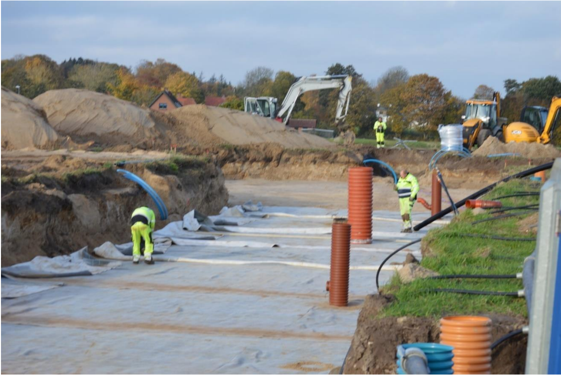
Figure 19. Construction workers placing bentonite mats at the bottom of the excavation pit. Eventually, bentonite membranes were placed on the excavation pit walls as well, creating a full seal of the roadbed, preventing seepage of groundwater into the roadbed.
