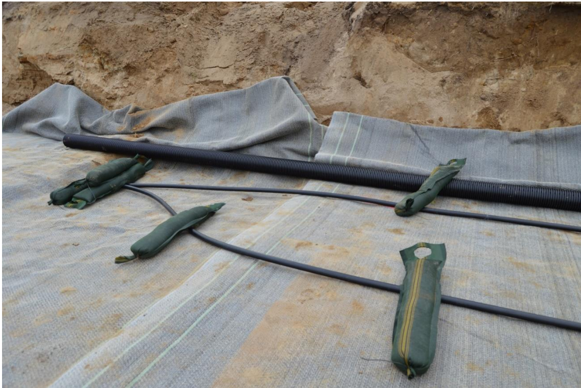
Figure 20. \varnothing 150 mm drainage pipe and a single \varnothing 40 mm SDR 11 U-pipe HE with a welded 180° bend.
