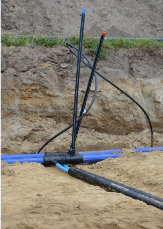
Figure 17. Connection pipes for the domestic heat pumps.
