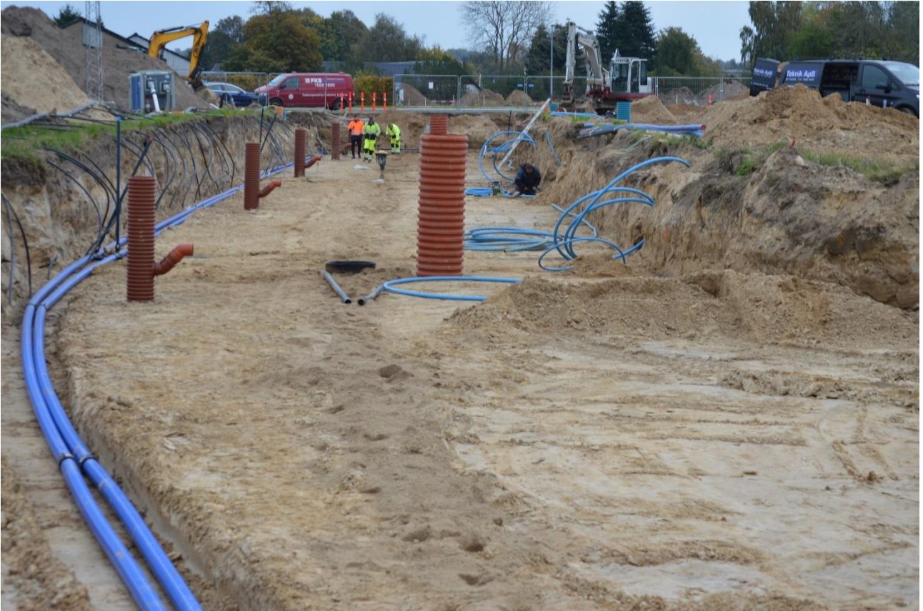
Figure 16. The roadbed excavation pit with uninsulated forward and return pipes in the left side of the picture. The black groundwater drainage pipes that keep the excavation from flooding, are visible at the left wall of the pit, near the distribution pipes.
