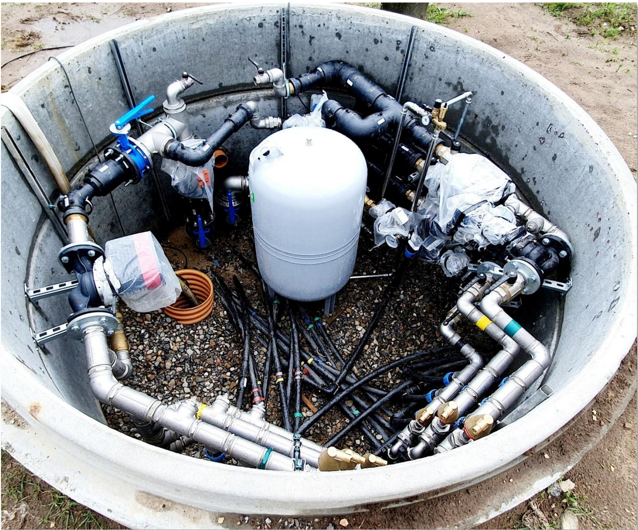
Figure 25. The Ø250 cm concrete manhole with geothermal piping, manifolds, dynamic valves, central pump, sump hole for seeping water removal, expansion vessel and energy and electricity meters. The Energy Machines control box for compilation of data and controls was not installed at the time the picture was taken.
